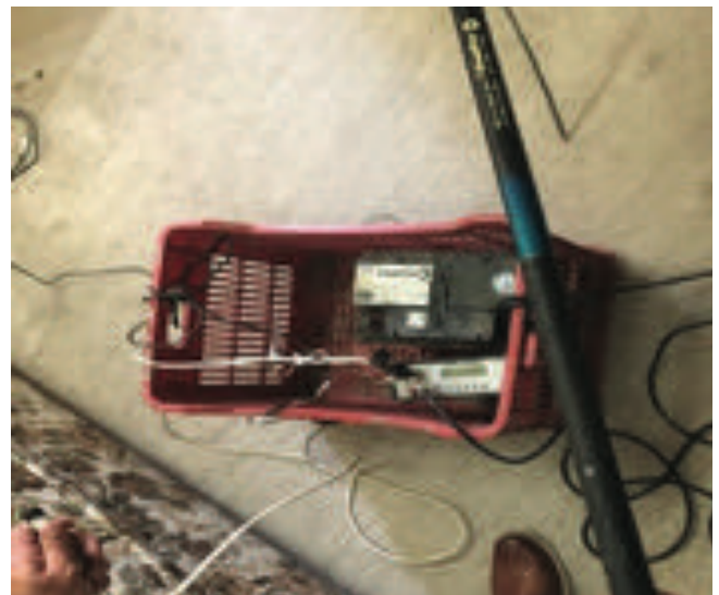
Figure 4. The improvised electrical installation.
